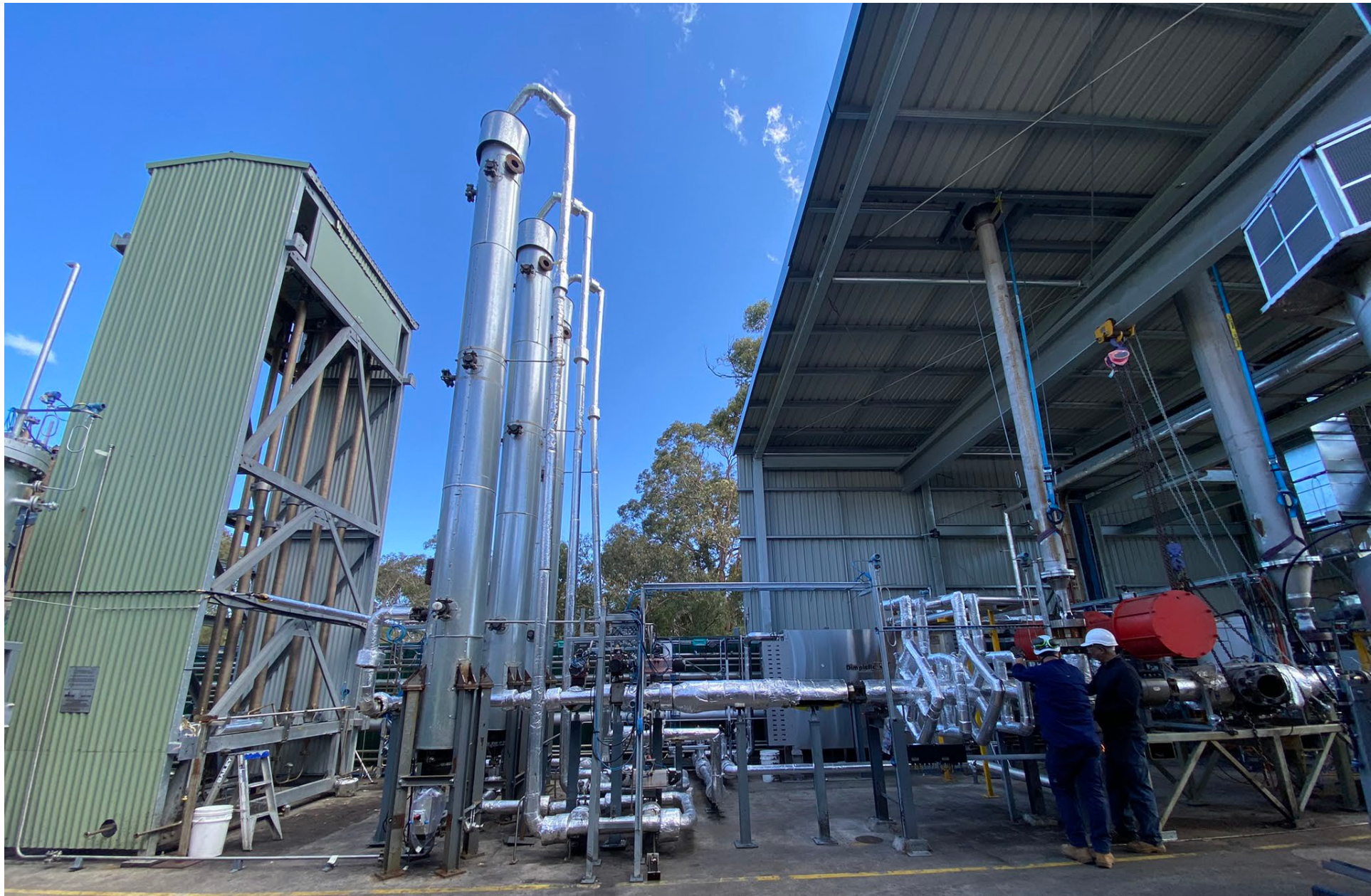
Licella's Cat-HTR™ Commercial Demonstration Facility in Somersby, NSW that converts biomass into biofuels.
